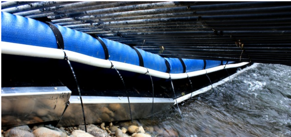
Figure 18. The Nisqually Weir air bladders filled with compressed air. Photo courtesy of Nisqually Indian Tribe.
